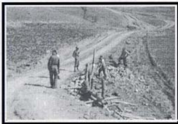
We widen Sprilla Road by filling it in with rocks at this narrow curve.
